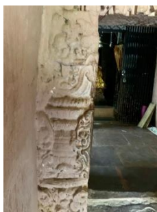
Photo 16: Left jamb of door-1
